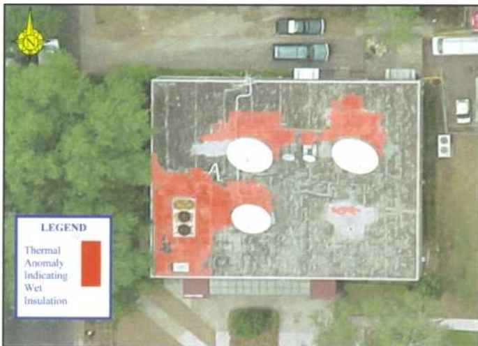
Note the hidden moisture caused by the poor installation of satellite dishes
